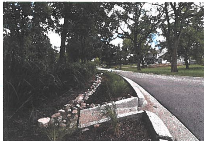
Curb cuts that drain to green infrastructure practices can be used as an alternative to traditional curbs and gutters.
