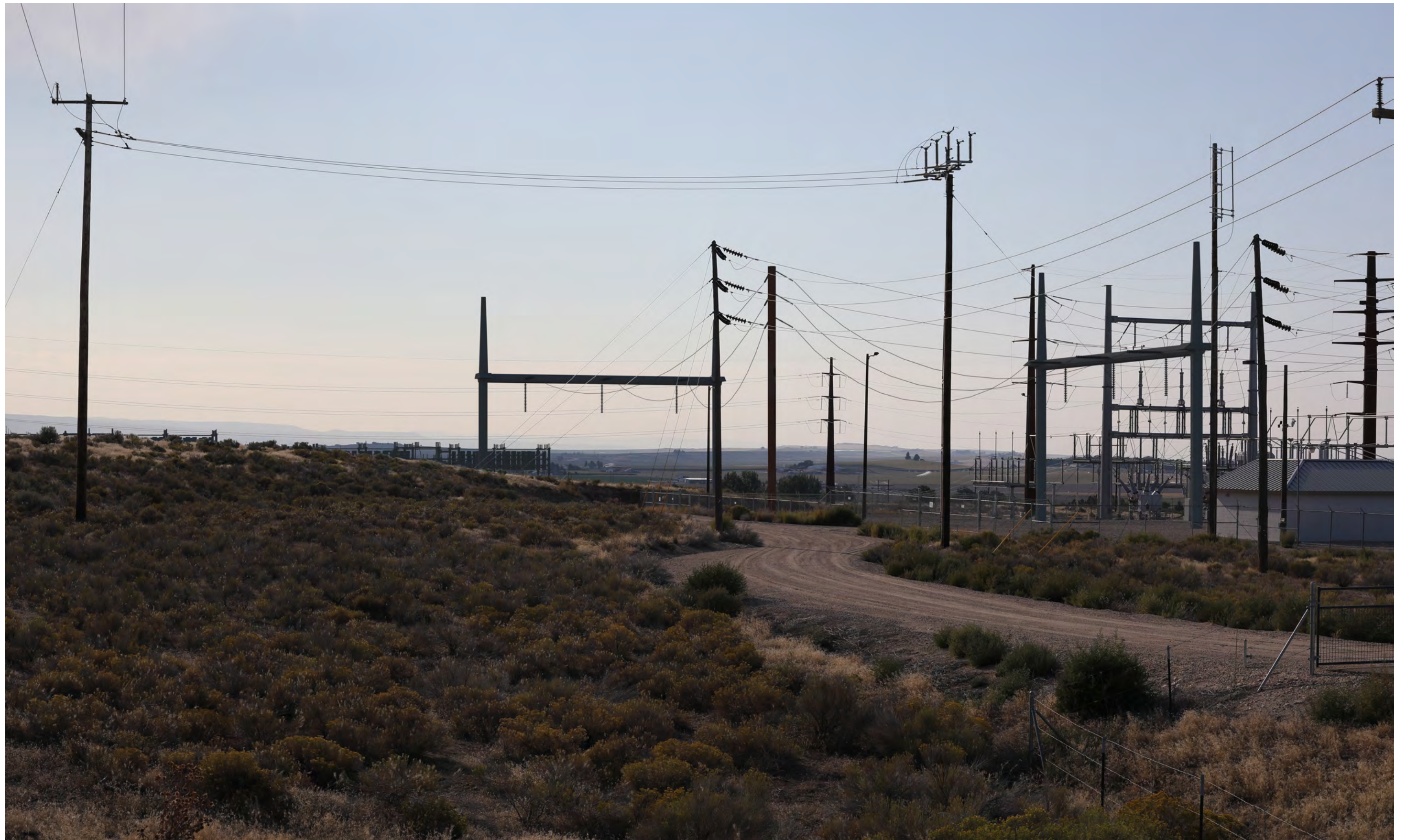
KOP 6: View from Intersection of Southside Boulevard and Rose Lane looking west - Simulated Condition
