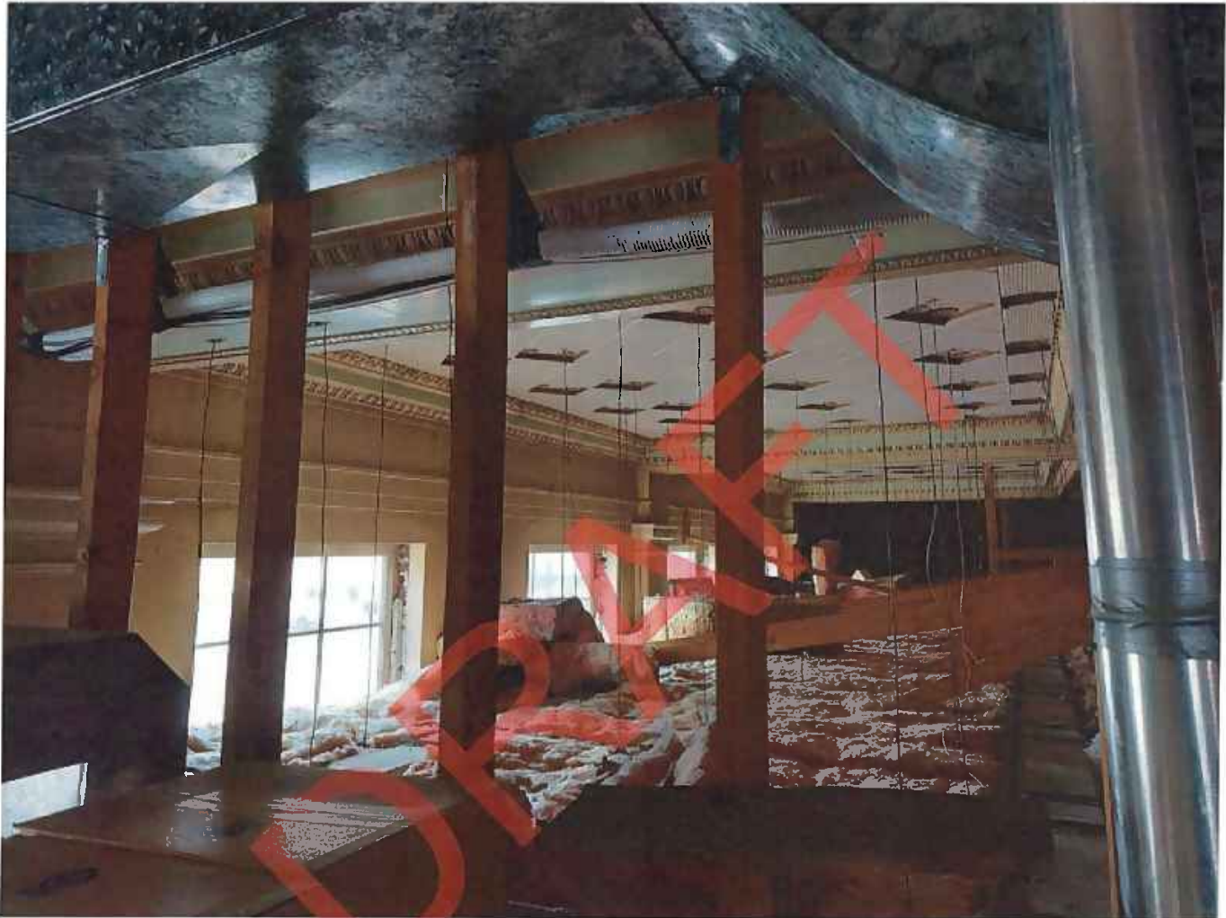
Photo 21 of 24. ID_Canyon_ParmaStateBank_0021 View above dropped ceiling along the north wall, camera facing northeast
