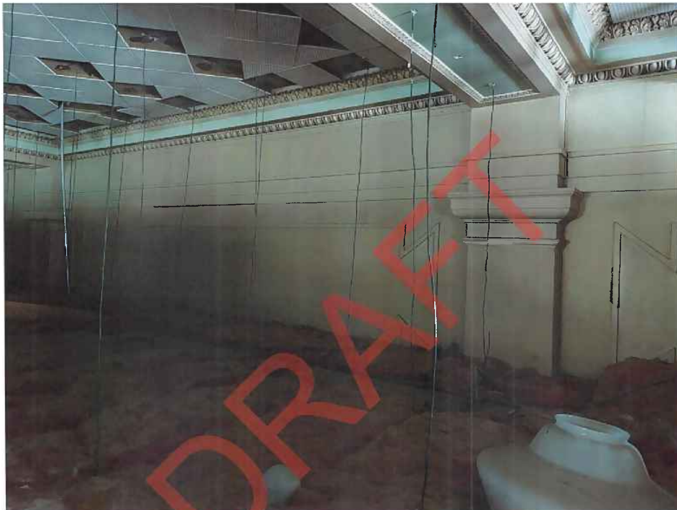
Photo 20 of 24. ID_Canyon_ParmaStateBank_0020 View of south wall above dropped ceiling, camera facing south
