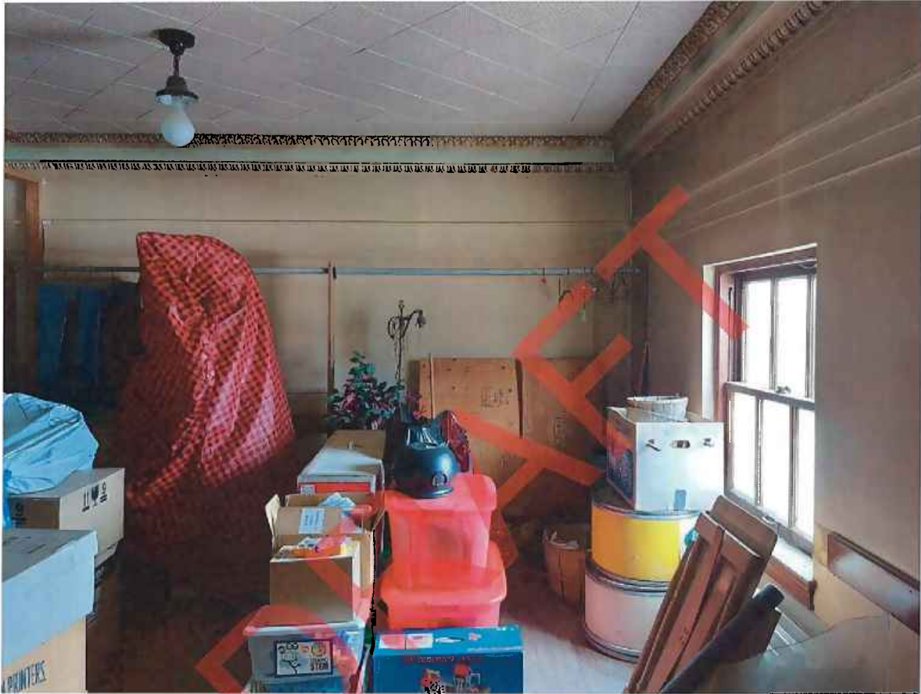
Photo 19 of 24. ID_Canyon_ParmaStateBank_0019 View of mezzanine level at the southwest corner, camera facing south
