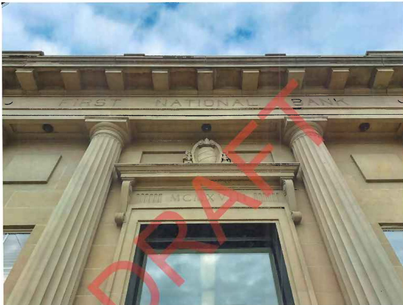
Photo 8 of 24. ID_Canyon_ParmaStateBank_0008 View of roofline detail on east (primary) façade, camera facing west
